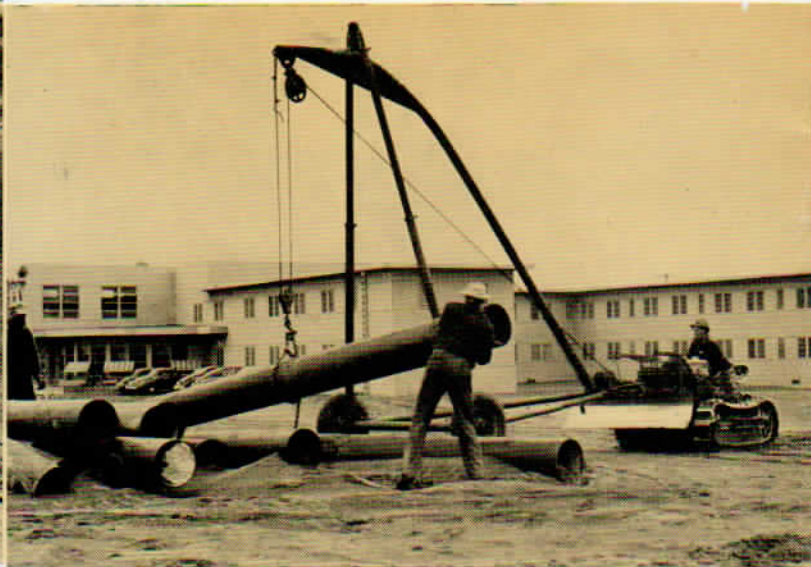
Upper right: When speed counted in Navy construction the Lindeman Tractor Crane was there to help.
